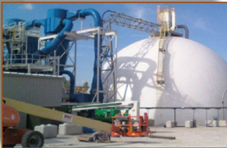
Limestone storage dome and conveyor equipment
